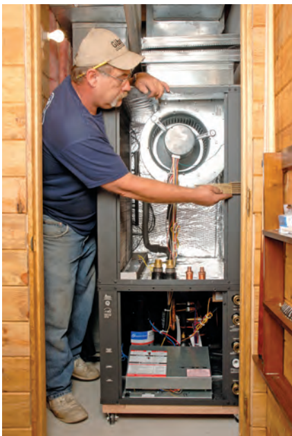
Scott Barnett works on the new ClimateMaster water-to-air heat pump, rated at 27-SEER. This unit provides all cooling and supplemental heat.
