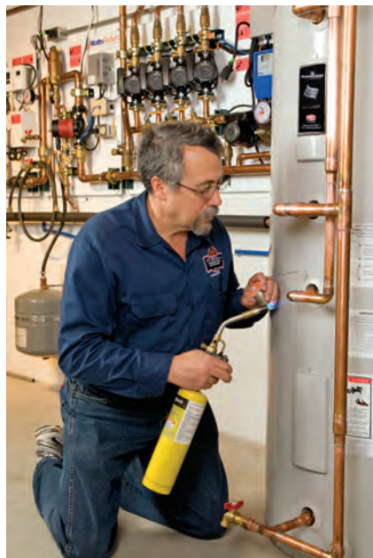
Dave Yates does final soldering on the buffer tank that connects to the hydronic control panels in the background.
