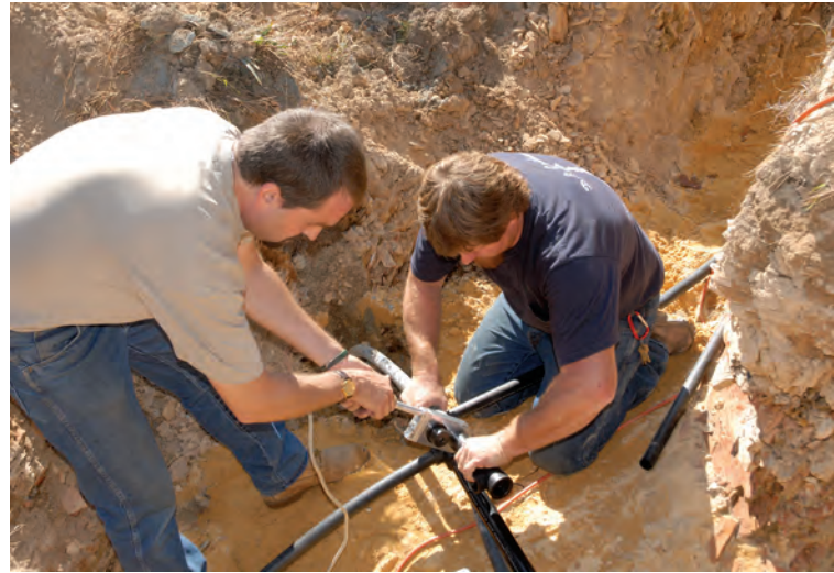
Fred Umble of Creative Energy (left) hot-fuses geothermal pipe connections at one of the three well-heads.
