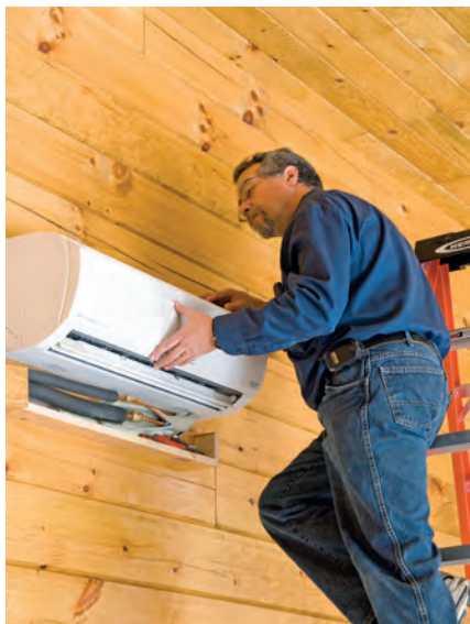
Dave Yates installs backup Fujitsu minisplit heat pumps, which also provide air-conditioning for interior garage spaces.
