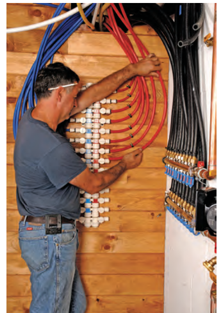
Travis’s father, Merv Wenger, installs the Sea Tech “home-run” domestic water lines into the central manifold.
