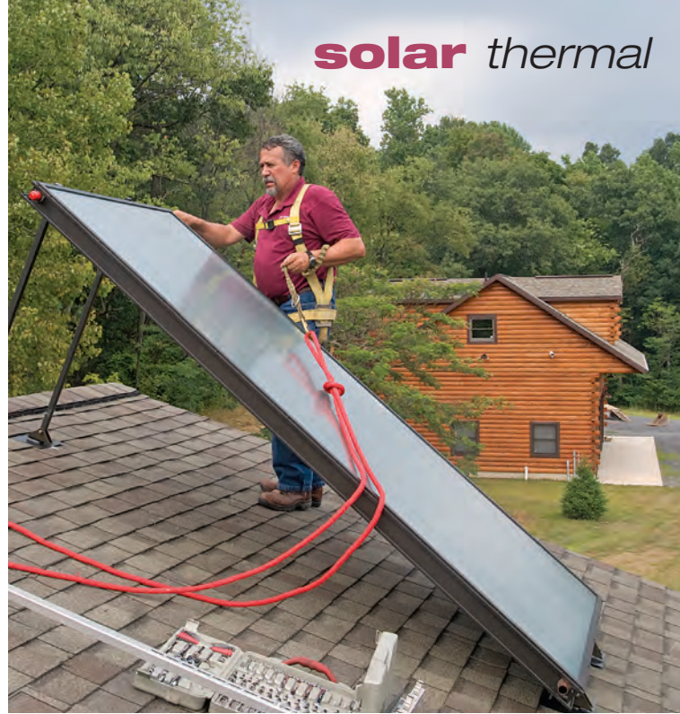
The Oventrop flat-plate collector is installed on the house's roof (the detached garage is in the background).
