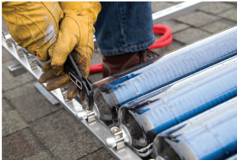
Clipping the bottom of the tubes into the lower end of the rack.
