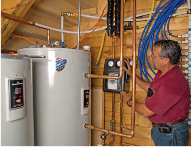
Storage tanks and pump-stack/controller.
